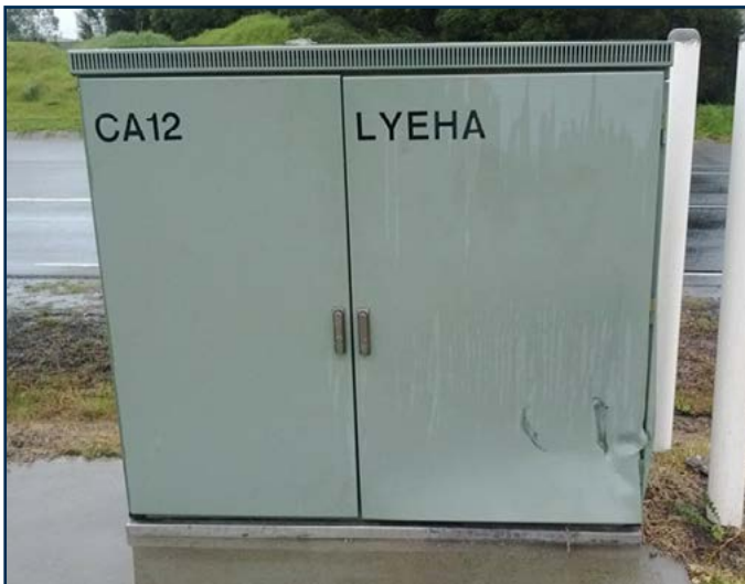
1. Damaged doors subframe and knocked 100mm out of plumb (leaning over)
