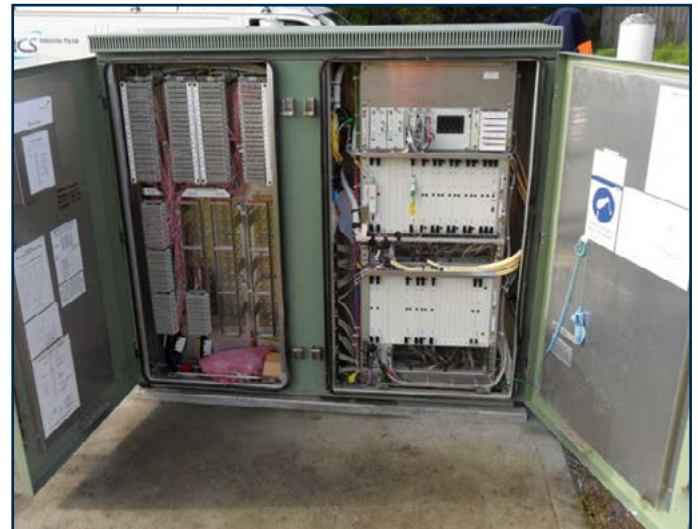
2. Damaged doors on cabinet leaning forward and stopping door from fully opening
